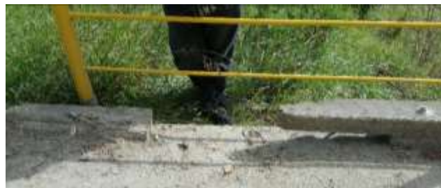
Figure 3: Bumper Pad to be replaced
