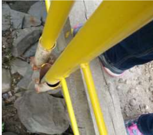
Figure 2: Sleeve needing repairs
